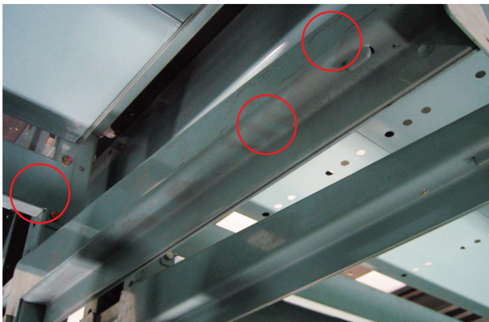
Figure 1. Racks with mould, dirt and rust. Photo courtesy of Alvin Tee
