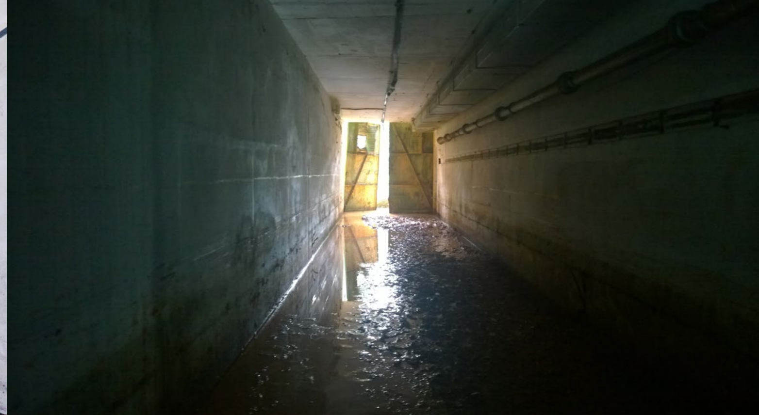
Flooding to the corridor to the bunker's entrance
