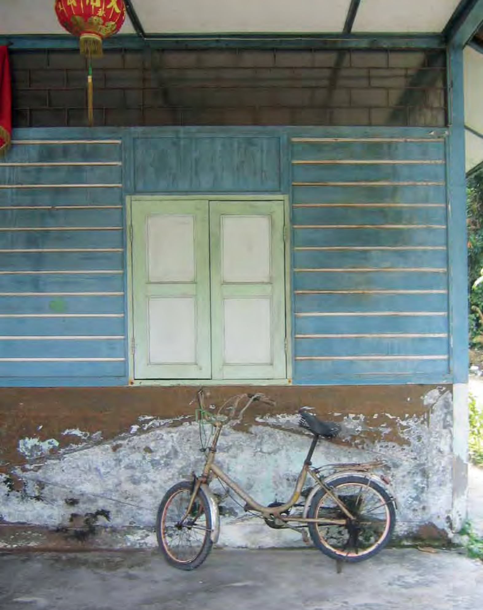
Close up showing the typical construction of a Chinese farm house. Picture is author's own.
