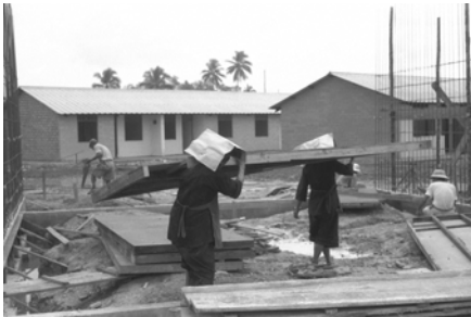
Samsui women working at a construction site in Toa Payoh, 1962 Ministry of Information and the Arts Collection, courtesy of National Archives of Singapore
