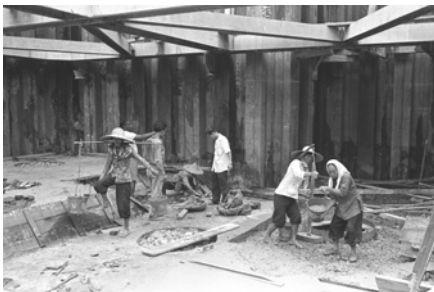
Construction workers working on a sewerage project in Toa Payoh, 1964 Ministry of Information and the Arts Collection, courtesy of National Archives of Singapore
