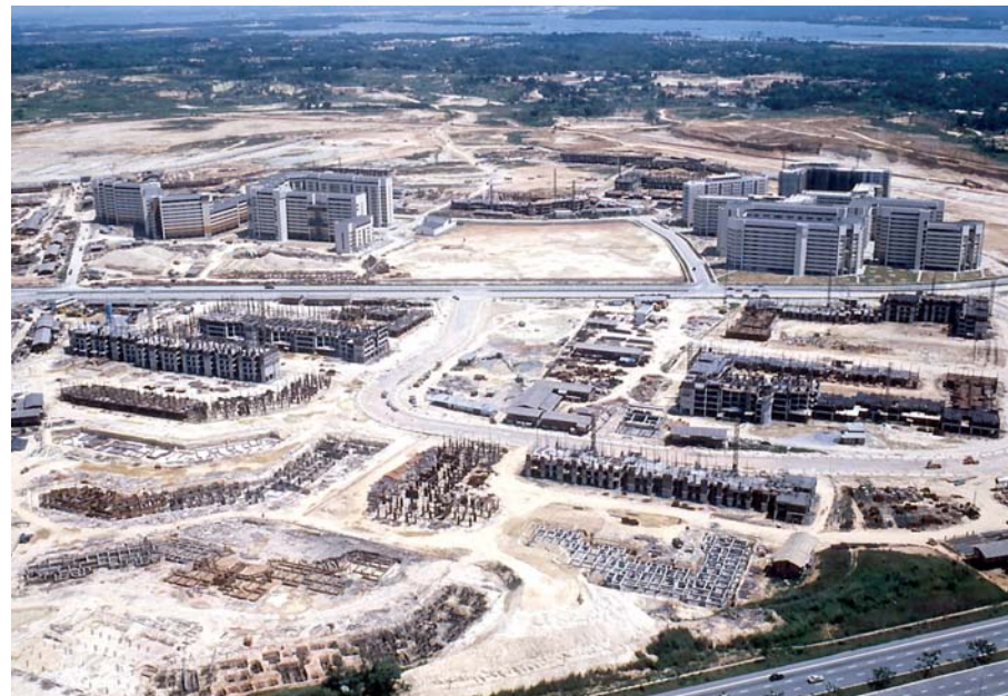
The construction of Tampines Town in progress, 1982 Courtesy of Housing & Development Board
