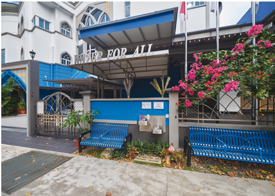
The water coolers installed for public use under Masjid Al-Istighfar's "Water for All" initiative, 2019 Courtesy of National Heritage Board
