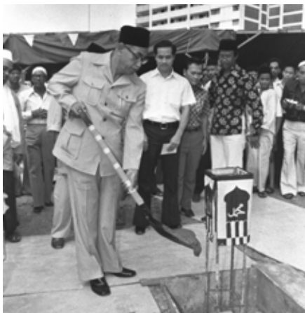
Syed Ali Redha Alsagoff performing ground-breaking ceremony for Masjid Al-Muttaqin, 1979 Masjid Al-Muttaqin Collection, courtesy of National Archives of Singapore
